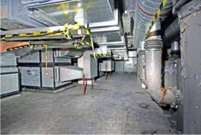
Air-conditioning plant room on the lower level
